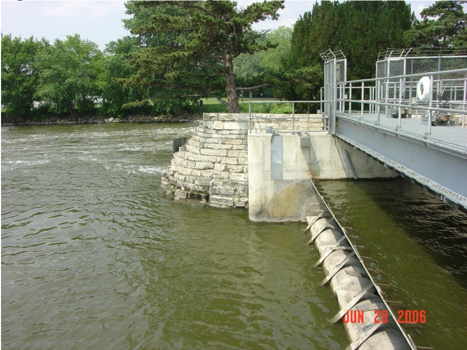
Figure 7: Stratton Dam Hinged Crest Gate
