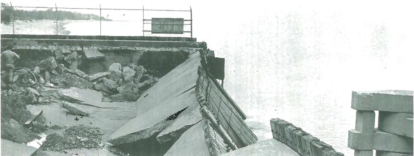
Seawall at Camp Logan damaged by wave action in November 1963.
