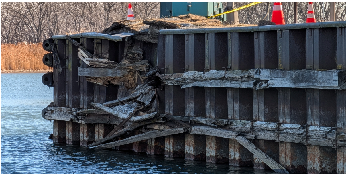
Figure 2: Damage to guide wall caused by barge impact.
