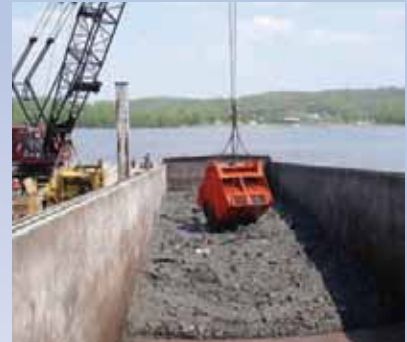
Loading barge on Lower Peoria Lake with sediment excavated with a clamshell bucket designed to minimize the amount of water placed in the barge.
