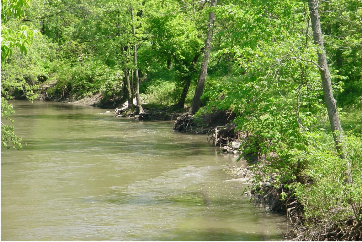
Figure 4. Longitudinal peaked stone toe protection and submerged riffle in high water on May 21, 2009.
