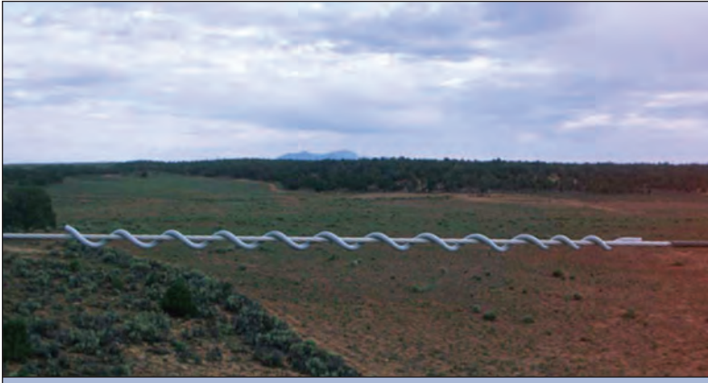
FIGURE 6.10: Spiral vibration dampers act to reduce line vibration, and they also make power lines more visible to birds.
