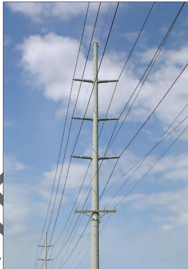
FIGURE 1.7: Distribution underbuild on a double-circuit transmission line.
