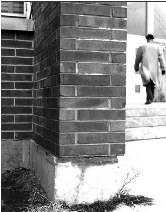
Figure 28 The largest movements are at the edges of the long, continuous wall. At this point, the short brick wall is being pushed off the foundation by the long, continuous brick wall to the left.
