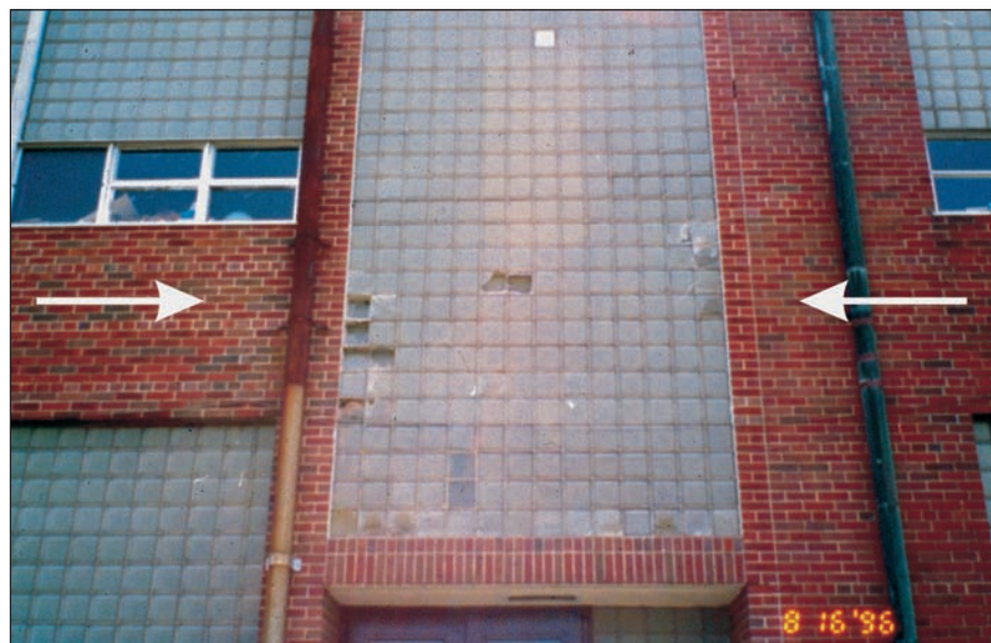
Figure 29 The long, continuous brickwork intersects the vertical glass block wall. Pressures have broken the glass blocks in line with the long, continuous expanse of brickwork.
