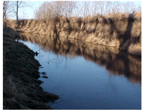
Figure 4. Unnamed tributary, north of 1100 N, looking upstream showing bank erosion and pooled water behind rock riffle grade control structure.
