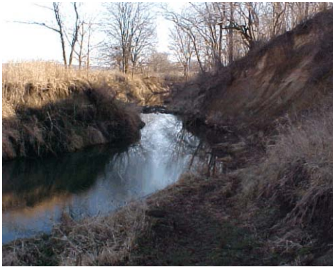
Figure 3. Unnamed tributary, north of 1100 N, looking downstream showing bank erosion and rock riffle grade control structure.
