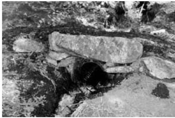
Figure 30--Culverts need to be installed at a sharp enough angle to prevent sediment from being deposited.
