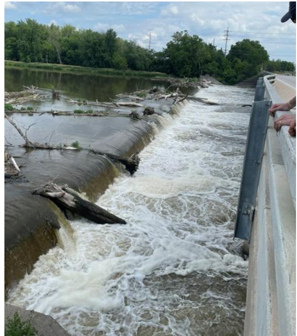
Figure 18: Sears Dam, looking from river right on Highway 67. June 13, 2024. 41.461637, -90.578965.
