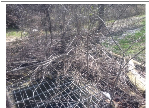
Figure 2.15 Detention basin outlet structure requiring maintenance
