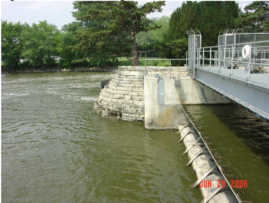
Figure 7: Stratton Dam Hinged Crest Gate
