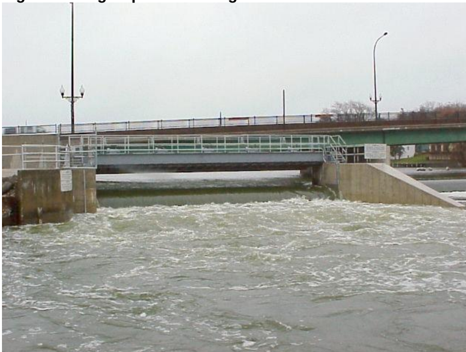
Figure 14: Algonquin Dam Hinged Crest Gate
