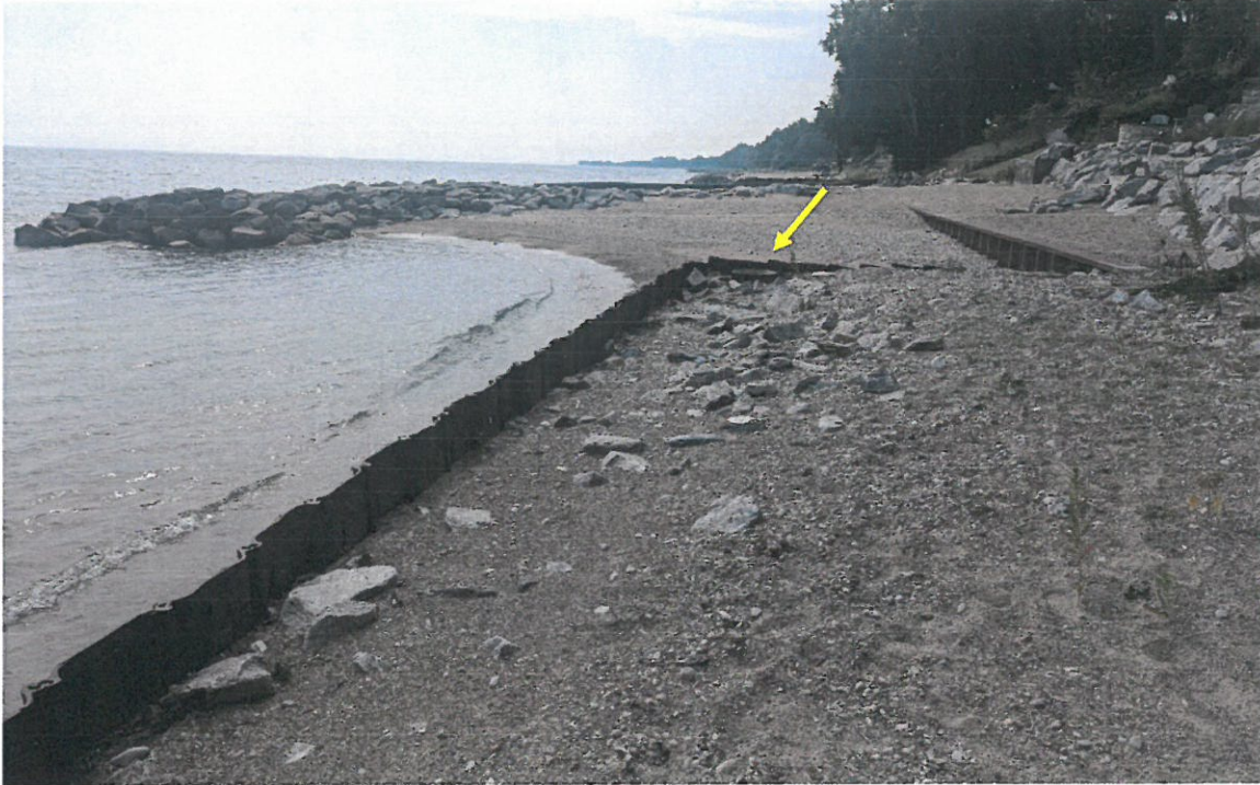
2025 Photo looking south shows existing seawall to be removed and existing stormwater outfall to be relocated west (yellow arrow)
