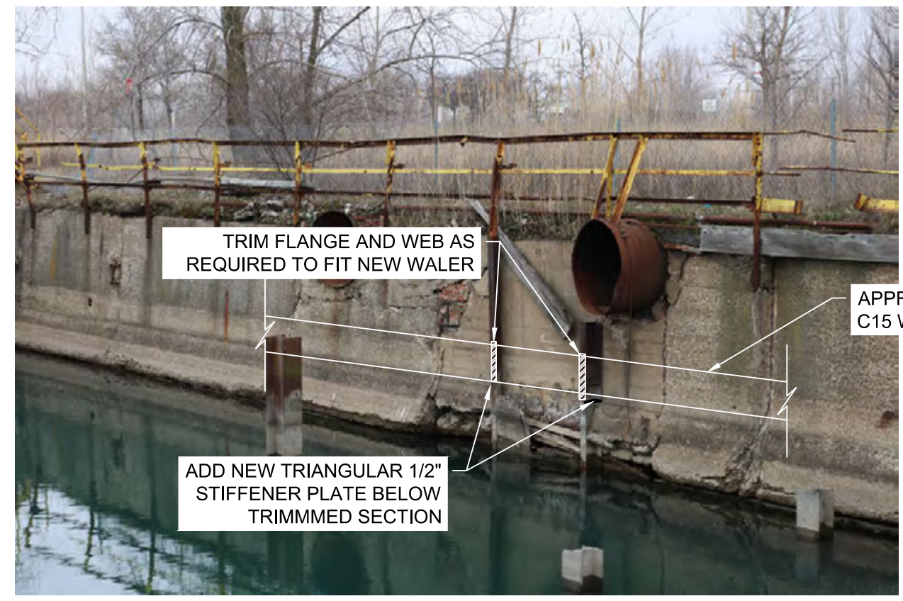
6 SECTION: EXISTING STEEL DEMOLITION ON WEST WALL NOT TO SCALE NOTE: 1. PHOTO TAKEN LOOKING SOUTHWEST.
