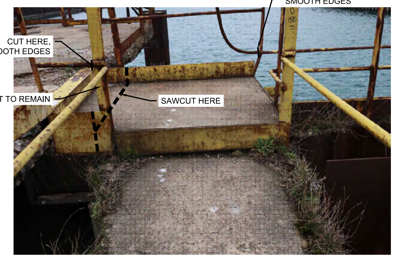
3 PHOTO: CENTER OF SLIP NOT TO SCALE NOTE: 1. PHOTO TAKEN LOOKING EAST.
