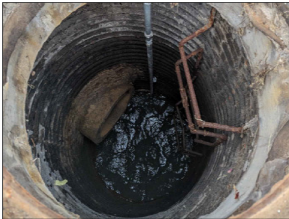
PHOTO: 14 DIRECTION: DOWN DATE TAKEN: 06-16-2023 NOTES: EX. SS MH5
