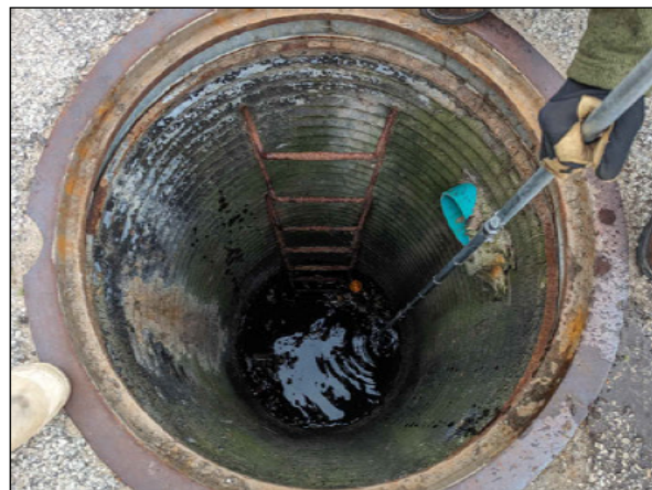
PHOTO: 5 DIRECTION: DOWN DATE TAKEN: 06-16-2023 NOTES: EX. SS MH 1
