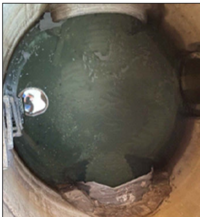
PHOTO: 15 DIRECTION: DOWN DATE TAKEN: 06-16-2023 NOTES: EX. SS MH5
