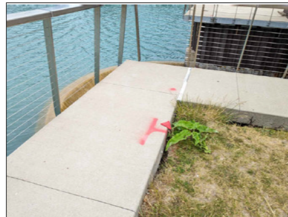
PHOTO: 7 DIRECTION: NORTH-EAST DATE TAKEN: 06-16-2023 NOTES: EX. HANDRAIL/ EROSION
