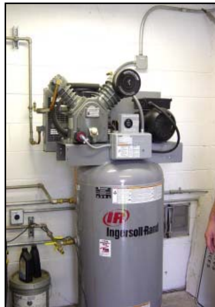
Obermeyer Gate Air Compressor in the Obermeyer Control Building
