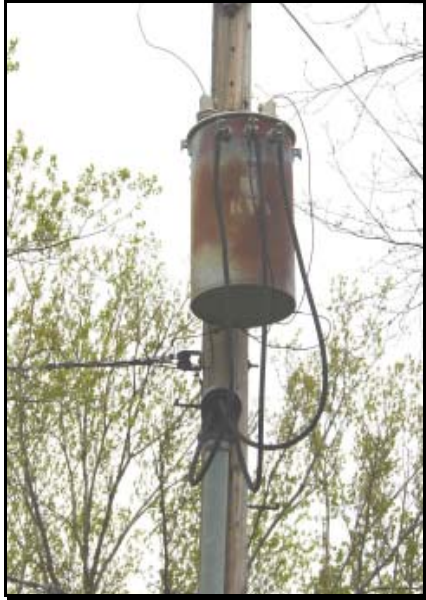
Power Utility 50 KVA Pole-Mounted Transformer
