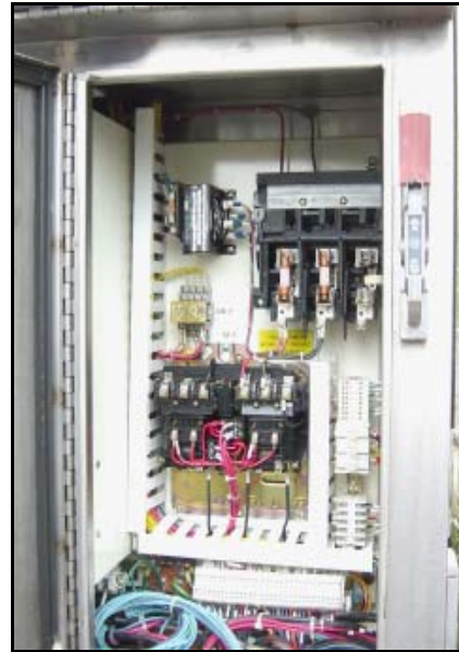
Reversing Contactors below the Mitre Gate Control Station
