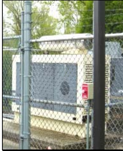
70 KW Standby Generator
