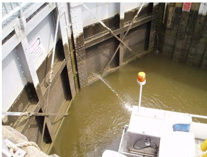
Small hole through the 3/8" steel skin plate
