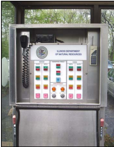
Mitre Gate Control Station
