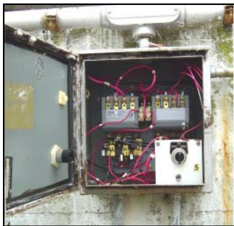
Sluice Gate Reversing Starter adjacent to each Actuator Motor
