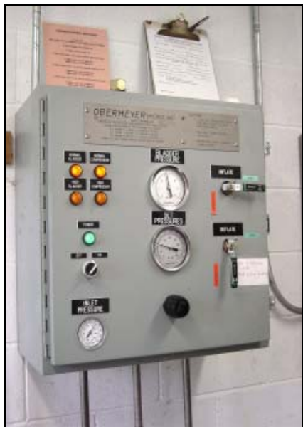
Obermeyer Gate Control Panel in the Obermeyer Control Building
